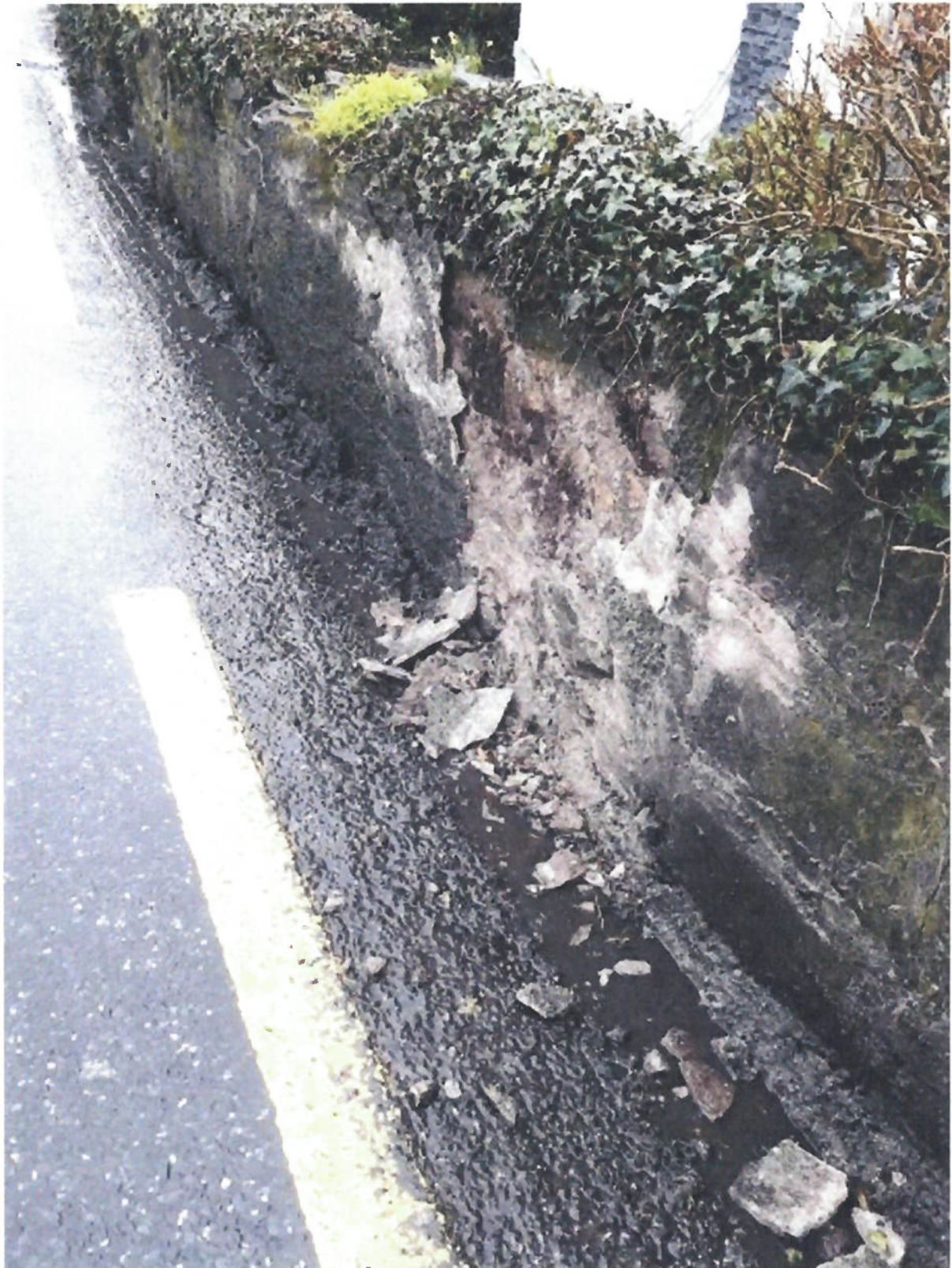
Front wall struck by an HGV 23/01/2019
